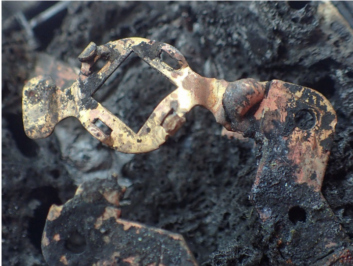
Photo 3: Welded contact points within a failed DC isolator
